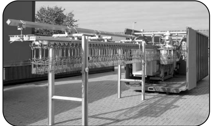
Mobile electrical waterbath stun/kill system
